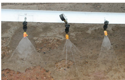
Spray Pattern is Off Due to Chipping and Cracking in Deflector
