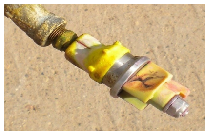
Cracking on Body of Nozzle
